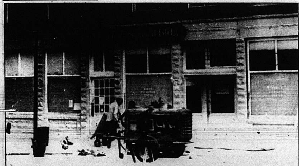
There was a lot of sandblasting going on at the Signal Building last weekend with James Anderkin and Bill Taylor doing the work. Best guess is that it is the first time the stone has been cleaned since the building was constructed in 1912-13.
