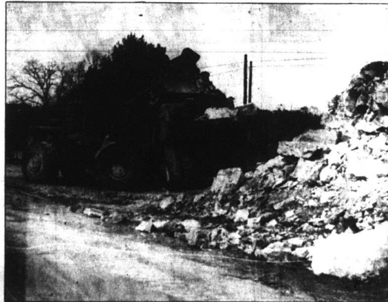
Construction of the intersection of U.S. 25 and the Mt. Vernon by-pass of 461 near Red Top Restaurant got underway Tuesday. But, the by-pass is not scheduled to be completed and open to the public until at least August.
