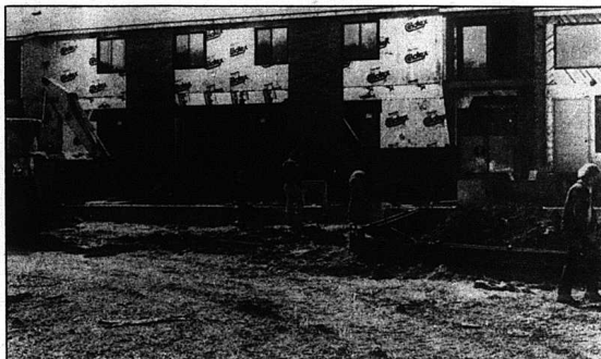
Work is progressing on a new apartment complex just off Tevis Street in Mt. Vernon near the Rockcastle Hospital. The complex, named Mt. Vernon Greens, is privately owned and developed by a Lansing, Michigan firm. No opening date has been reported. For further information telephone 256-2507.
