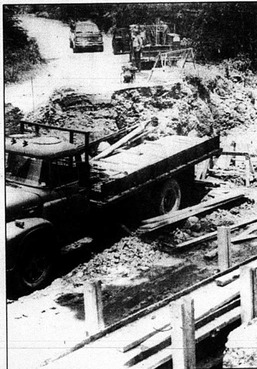
Workers for Polly and Trent Construction Company of Bardston is replacing a bridge on the Brodhead/Chestnut Ridge Road at a cost of $69,976. The bridge is expected to be completed this fall.
