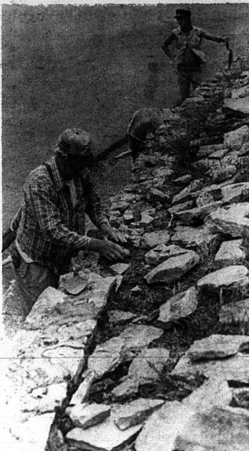
Elmwood Cemetery wall in Mt. Vernon is getting a new cap, the first since the wall was constructed by the Jaycees in 1970. Doing the work above are Andrew Miller, contractor, and Marshall Cameron, Henry Cox, a cemetery director, said time and vandalism had eroded the top layer of the wall.
