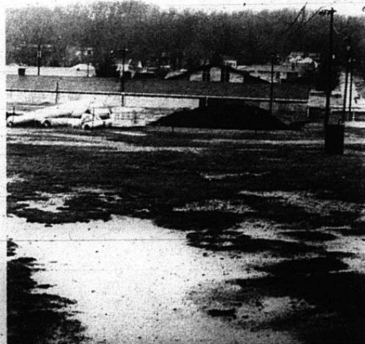
Excavation has already begun at the new Mt. Vernon Elementary School construction site. Work has been slowed by a wet winter.
