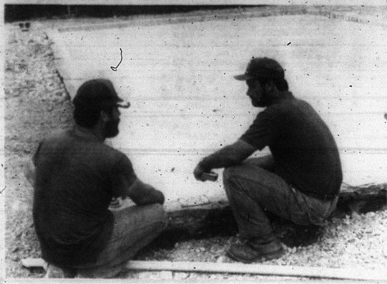
Jerry Fritz, right, who oversees all construction and maintenance at the new Renfro Valley complex, discusses the renovation of the swimming pool with James Flannery. The pool, which is expected to re-open this month, will include a wading pool shaped like a guitar, a shower room and a game room. The bottom of the pool will be painted with musical designs. Many changes are taking place in the valley at the present time. Earlier this year the complex was sold to investors, who have also purchased the Renfro Valley Lodge and Restaurant, a drive-in restaurant owned by Mr. and Mrs. Joe Allen and several acres of land owned by Bill Davis. (Photo by Herb Sparrow)
