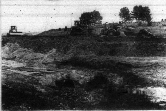
Work is now underway on KY 461, where excavation is less than a half-mile from Wabd.
