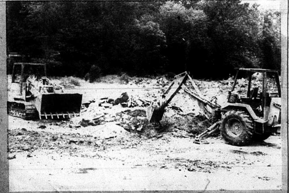
Workers have been clearing the old Belly Acres Restaurant property at Exit 62 off-75 on US 25. The owners say the property is not for sale.
