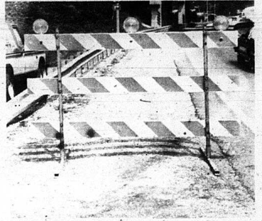
Barricades like the one above have been moved from the new 461, which causes concern for the contractor about the safety of those traveling along old 461.
