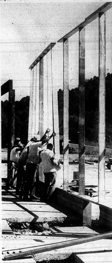
Workmen put up the frame for one wall of the planned saw mill at the new Mt. Vernon Hardwoods east of the city. The mill, which will be capable of sawing furniture grade-wood to be shipped to a Burnside factory, should be in operation in mid-October. Right now, the company is buying logs. When in full operation, the mill will hire 12, and could add to that number later.
