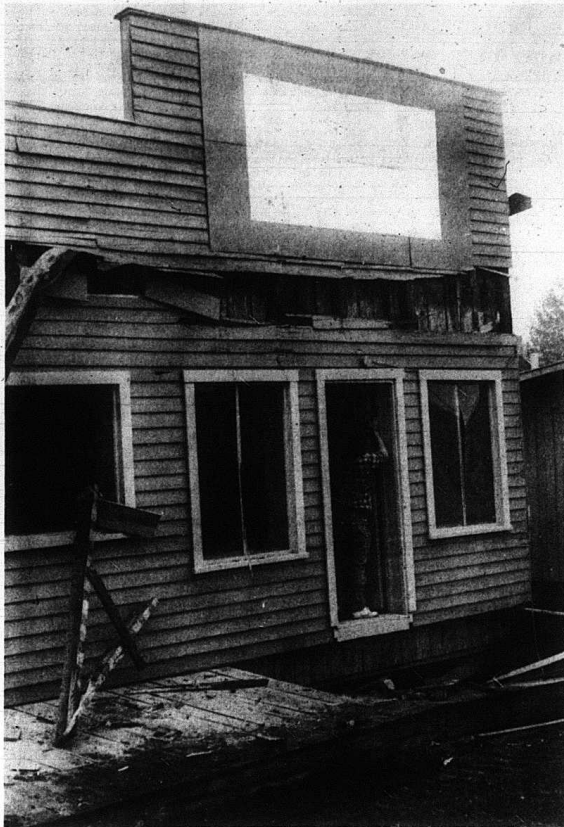
Workers were busy last week demolishing Old Main Street in the Valley (with the exception of the former home of Log Cabin Crafts which is being moved into Renfro Village). Local residents got quite a shock Thursday night when it looked as though everything at Renfro was burning down. But, as those who inspired found out, it was a controlled burn by the Mt. Vernon Fire Department of all the debris from the demolition.
