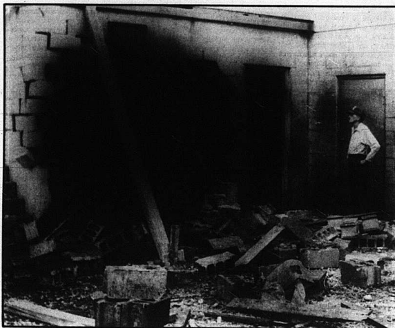
Brodhead Mayor Billy Bussell views the remains of the boiler room at the rear of the city hall building that was destroyed when the boiler exploded Sunday.
