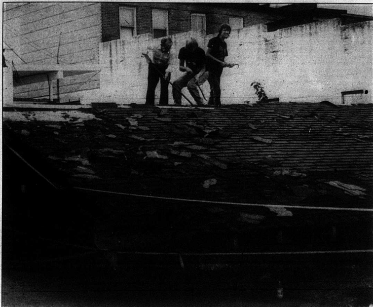
Edward Deborde, Ricky and Ronnie Barnett work on the roof of the old building that was once the clothing store of Mary Ida Jones. The area will become a parking lot for Bank of Mt. Vernon employees.
