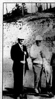
Groundbreaking at the site of a new sewer line through Renfro Valley was held Tuesday. Attending were, from left: County Judge/Executive Roland Mullins; Harlan Kenny, contractor; Ralph Gabbard, president RenfroFolks, Inc.; B.J. Ewen of Nesbitt Engineering; Mt. Vernon Mayor Gary Cromer; Paul Nesbitt of Nesbitt Engineering; Attorney John
