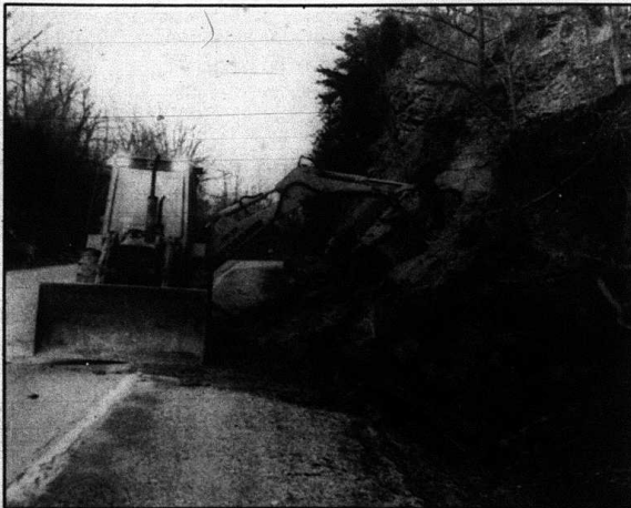
Workers were busy Tuesday and Wednesday trying to clean the debris from a rock slide in the gap on U.S. 25, just south of Mt. Vernon. One lane of the road was completely blocked during the clean-up effort.
