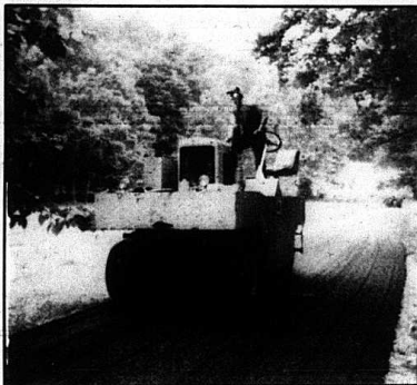
New blacktop is rolled on Kings Hollow Road, one of many being upgraded by the county.
