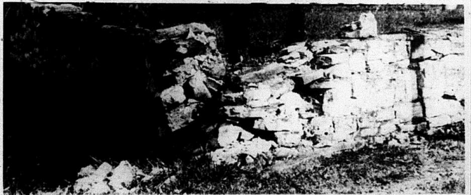
Broken Down Walls
