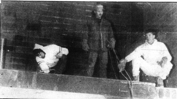
Workers were busy last week placing steel beams in what will eventually be the new gym at the new Rockcastle County High School. Local school finance officer Richard Bray, who is overseeing the project, told the Rockcastle County Board of Education Tuesday night, that project was on schedule opening in the fall. (Photo By: Richard Anderkin)
