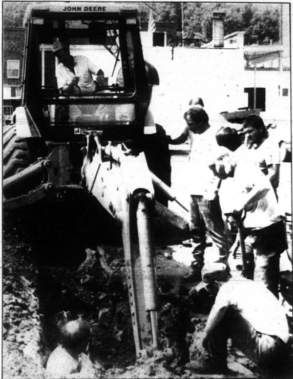
City of Mt. Vernon water and sewer employees and local contractors Dexter Roberts were busy Tuesday laying a new sewer line for the RTEC building on main in Mt. Vernon. The job was finished in one day and will keep the sewer from backing up in the RTEC building. The sewer had been traveling uphill.
