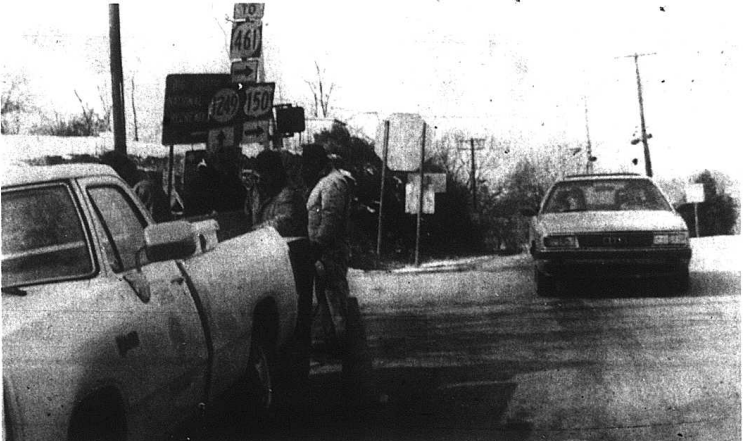
State transportation workers have been working in Mt. Vernon for a couple of weeks installing a four-way traffic light at the intersection of Richmond Street Hwy, 150, and U.S. 25 and Town Hill road. Workers said Tuesday that the light should be in operation as early as next week.
