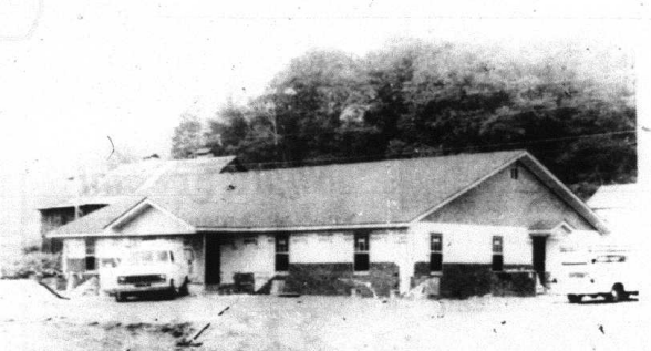
The local Farm Services Agency and Natural Resources Conservation Service will move their offices to a new location on Hwy. 150 between Mt. Vernon and Brodhead. The move is slated for October 1 to the new building being constructed by Benton Bullock.
