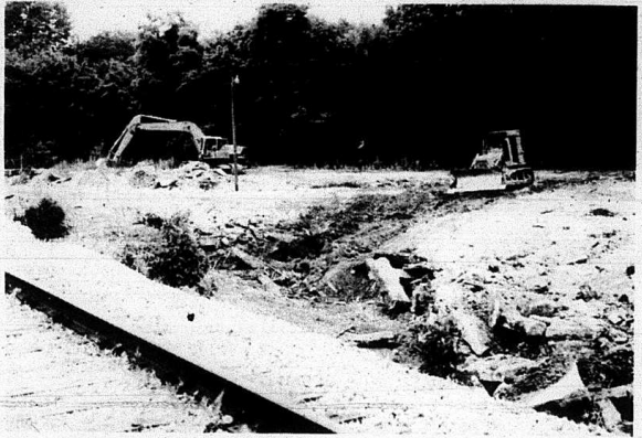
The City of Mt. Vernon has started clearing the site for the new city park which will be located on the former Thrifty Lumber Company property on Williams St. in Mt. Vernon
