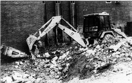
Work has begun on the new addition at the Rockcastle County jail. The building project, which will cost an estimated $900,000, will add 28 beds for prisoners and will bring the jail in full compliance with state regulations for the first time in many years. The project is slated to be finished sometime late next year. Chris Goff of Goff Construction is shown moving dirt and rock from beside the courthouse for the new construction phase of the project.
