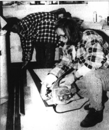
Etta Edmonson and Ida Brown worked at the Ashlee House Monday morning. A class sponsored by the Kentucky River Foothills Foundation has helped to remodel the local homeless shelter.
