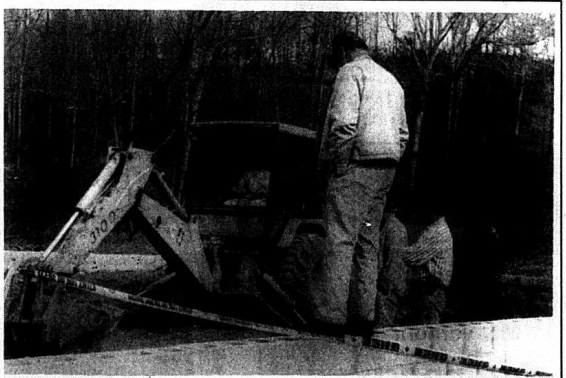
Rockcastle Sheriff Shirley Smith, Deputy Darrell Doan, KSP Detective Gary Lane and Jackie Goff, watch as Jackie Goff, uses a backhoe to move the muddy dirt inside a new housing footer on Tark Hill Road. Police had received a tip that Charles "Toddy" Baker was buried there, but they found only a toboggan.
