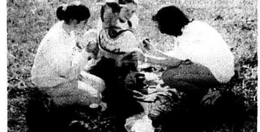
RCHS Y-Club members Ashley Lawson, Lyndsay Parsons, and April Martin working on the playground equipment they repaired and painted at the park.
