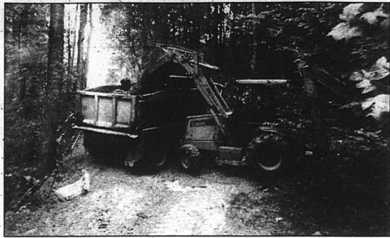
The Rockcastle County Road Department cleaned up a dumpsite on Vanzant Road near Burr last week. The dumpsite cleanup cost the county $1,572. Work release prisoners from the county jail also helped out. The county has also identified two different waste tire dumpsites. The smaller tire dump was located on Exit 62 within a few hundred yards of the interstate ramp and had 341 tires in it. The second tire dump was located near Buffalo, off the Sand Springs Road and contained approximately 3,000 tires. The county had only enough funds to dispose of 484 tires from the second dump, but were able to completely cleanup the first dump. The county will apply for federal funds to help pay for the cleanup at the second dump. Waste tire dumps are prohibited on public or private property by state law.
