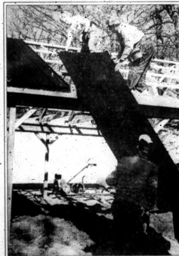
Joby McFerron hands up metal roofing for outdoor classroom made possible by a grant from PRIDE.
