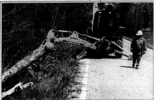
Kentucky Department of Transportation employees were busy Monday working to clear debris from the right-of-way on Hwy. 70 after a Sunday storm. Shown above are state road workers Paul Mason and Darrel Dillingham. Dillingham said that it appeared that a small tornado went through the Quail area around 7:30 a.m. Sunday.
