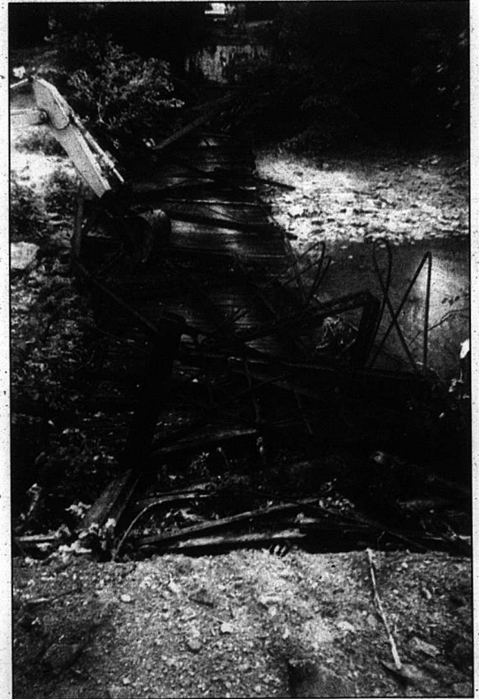
N & N Construction of Mt. Vernon is currently replacing the bridge on Mullins Station Road. The old, wood-dressed bridge was constructed in 1912. Work is expected to be completed in middle August.
