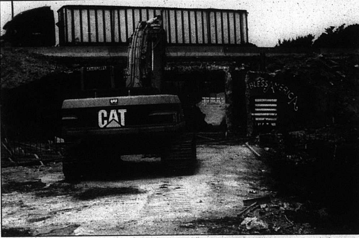
Flat Gap Road in northern Rockcastle County is currently closed because of construction on Interstate 75. Work crews are constructing a new bridge to include a third lane of the interstate. The road is expected to be open by the start of school in August.
