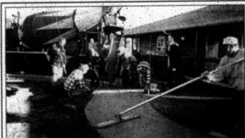
Installing a cement around a pond are Hank Gates, Don Huisenga, Hank Loerop, Roger Ellens, Rich Brouwer and Ken Ipema.
