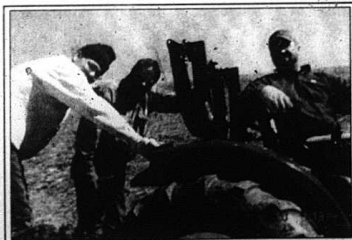
Mike Poppema, Larry Ribbens and Mike Kleinhesselink building a retaining wall around the greenhouse.
