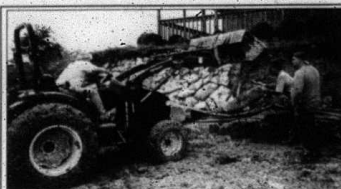
Hank Gate, Rob Van Riessen and Chris Ver Mulm building a rock wall.
