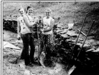
Emily Bosma, Jess Steenwyk and Holly Hoolsma digging a trench for wiring of greenhouse.
