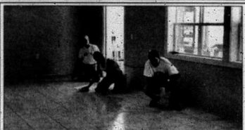
Alan Jewel, Tommy and Will came from Dalton Ga. to lay the tile.
