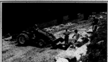
Hank Gates, Lance Barnes, Ron Bader and John Lindvall working on a rock wall.
