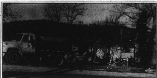
Clean-up work on the site of the former Casper Williams' home which was located on Main Street in Mt. Vernon for over 100 years, began this week. Wayne Carpenter's Construction Company is doing the work. The historic home and hotel, burned down over two weeks ago.
