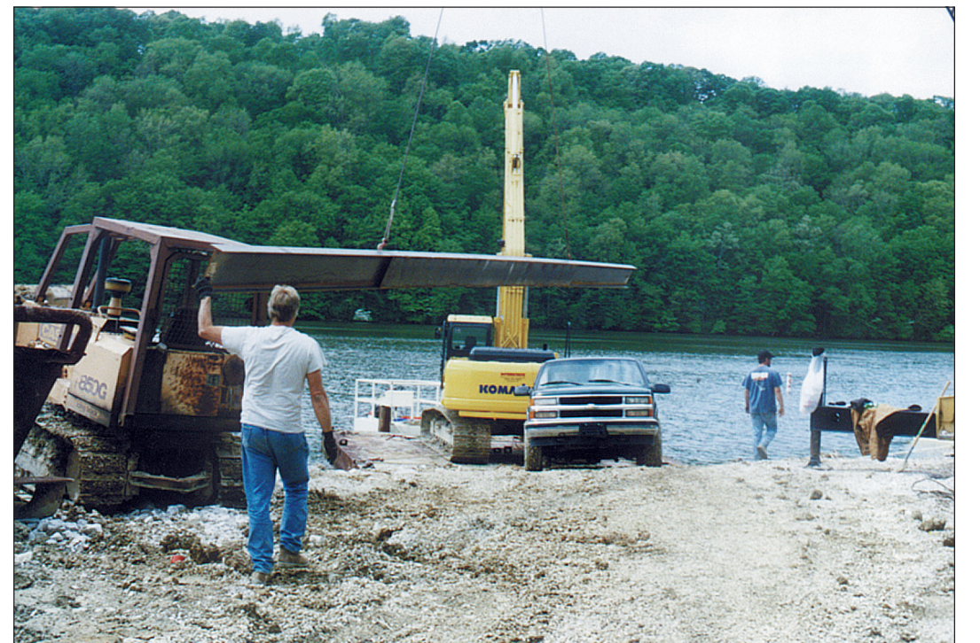
Work on improvements to the Mt. Vernon Water system has begun. Laurel Construction was the low bidder on Phase One of the improvement project at a price tag of $2.55 million. The project will add three new intake lines from Lake Linville to the water plant and there will also be seven different chemical lines added. Once completed, 6 million gallons of water will be able to be sent to the water plant although the plant itself can only process 4 million gallons a day at present. Water plant personnel will also be able monitor the quality of the water from the three lines, which will be at different elevations for the best quality. The city received a $1 million grant for Phase One of the improvements and are selling bonds for the additional $1.55 million. The city is also seeking loans and grants for Phase II which will include new water tanks and new lines to the tanks. Dale Lamb of Laurel Construction is shown helping unload a crane and materials for the project, which will take three to four months to complete, according to Mt. Vernon Mayor Clarice Kirby.
