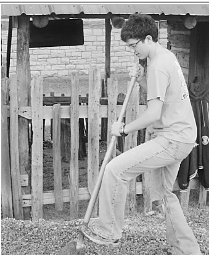
Senior trombone player Drew Davidson shovels gravel for the seating area of the cabins.
