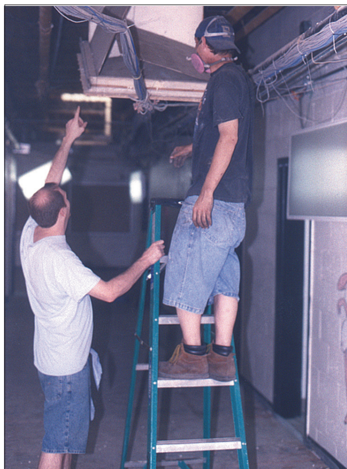
Work has begun on the new heating and cooling system at Roundstone Elementary School. Before the new system can be put in place this summer asbestos has to be removed from the school. Rockcastle County School's Building and Grounds Director Doug Mullins said that he anticipated the work to be finished by the beginning of the new school year on August 9th. Above, Max Combs, left, and Jeff Wolfe, work to remove asbestos from the school's ceiling on Tuesday.
