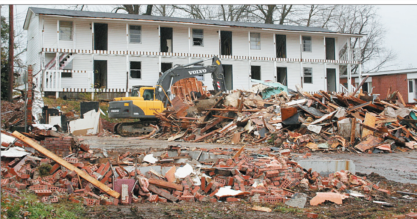
Clifford Collins, owner of Clifford Collins Backhoe LLC of Mt. Vernon, and Sam Stallworth were busy on Thursday tearing down the Northside Apartment structures on Richmond Street in Mt. Vernon. The site, along with adjoining property owned by Roger Isaacs, will be completely cleared in a few weeks. The property is owned by the Rockcastle County Industrial Development Board and totals approximately 1.3 acres. Industrial Authority Board Chairman Corey Craig said the house on the Isaacs property would probably be destroyed by a controlled fire set by the fire department.
