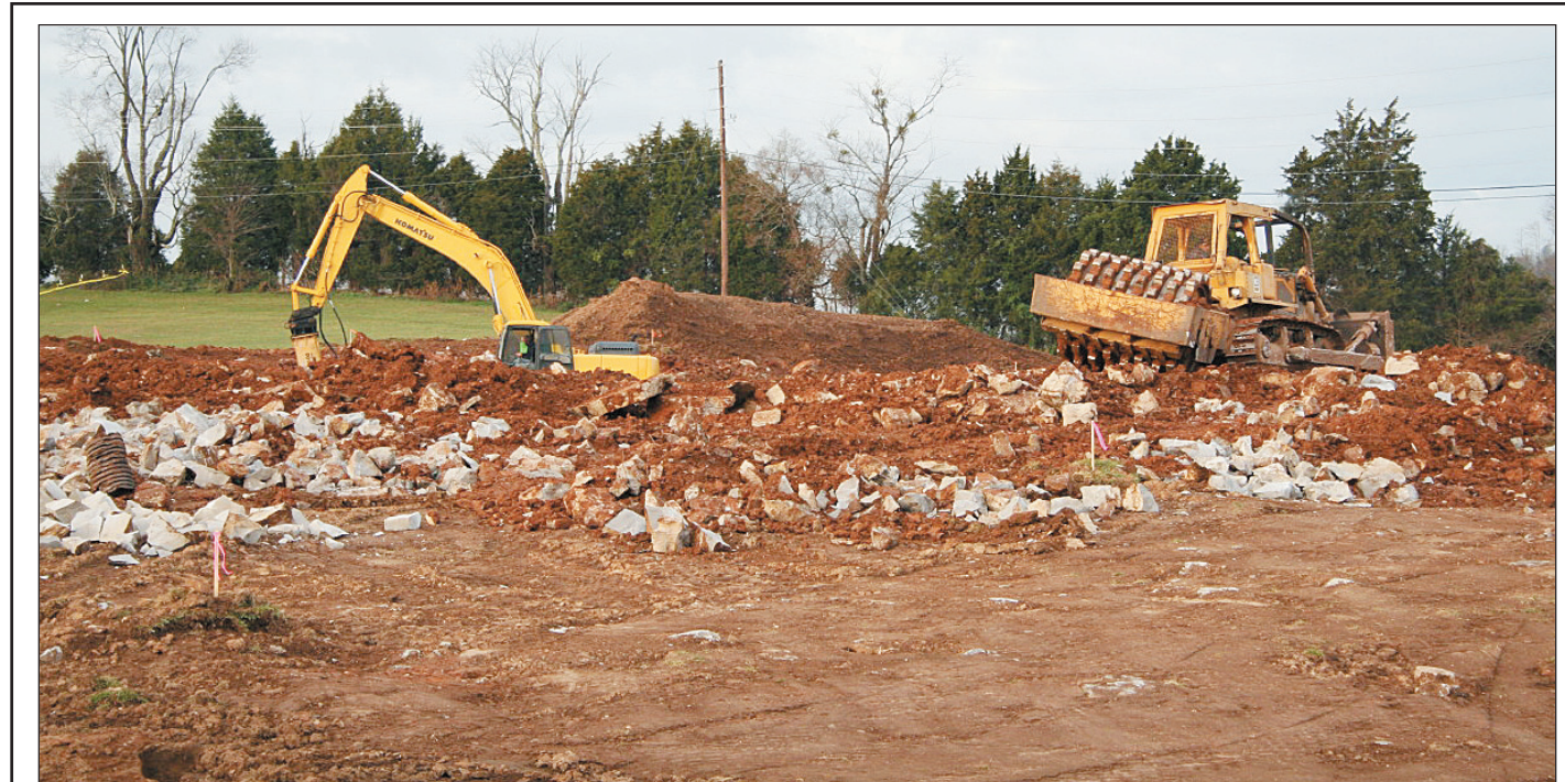
Construction has begun on the new $8.5 million Rockcastle Area Technology Center, which will be located adjacent to the Rockcastle County High School. For the past two weeks, employees with Goff Excavating of Brodhead have been preparing the construction site. The new building, which will be connected to the high school by a corridor, is scheduled to be completed by the start of the 2007-08 school year.
