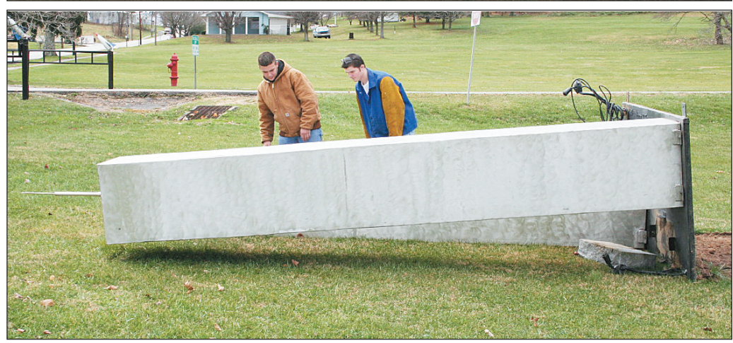
Heavy winds Friday caused problems for some people, including employees of D.W. Wilburn Construction Company. Employees are shown in the top photo trying to right a tool trailer that was blown over Friday morning at the construction site of the new Rockcastle Area Technology Center at Rockcastle County High School. Above, Curtis Burton and Jake Renner, students at the current RATC examine the damage to the replica of the Twin Towers, which were also blown over by the high winds. The towers were built by students in the welding program at the Technology Center as a memorial of the tragic events of 9/11. The towers were slightly damaged by the fall but are back on their "feet", once again.
