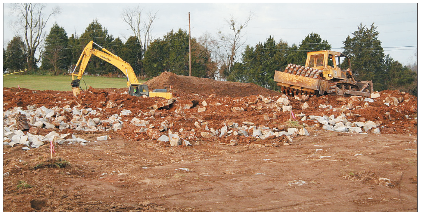
In November site preparation for the new $9.5 million Rockcastle Area Technology Center got underway beside the Rockcastle County High School.
