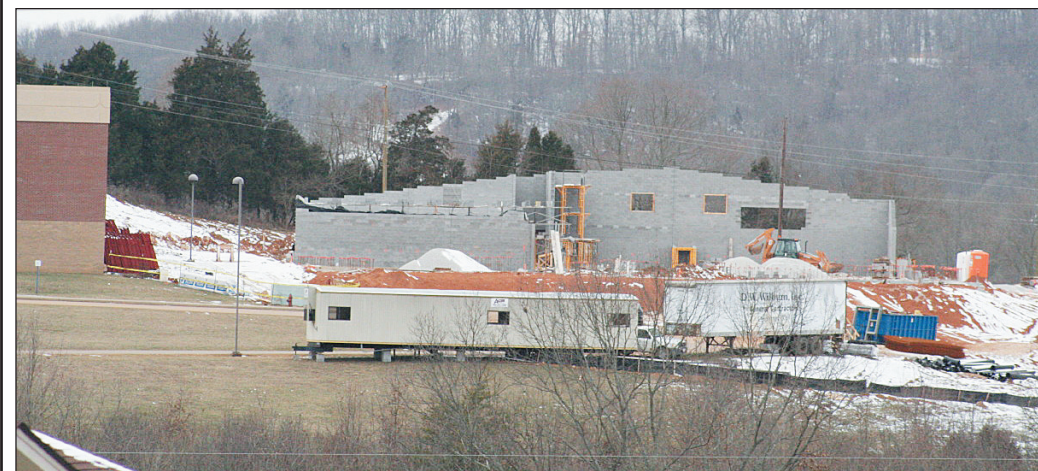
Even though it is winter time in the county, construction is going at two different school sites in the county. In the top photo is the new gymnasium at Roundstone School which is on schedule to be completed by April 19th. The cost of the new gymnasium is approximately $1.5 million. On Monday, Building and Grounds Director Doug Mullins was on site to inspect the progress. In the bottom photo, work is also well underway on the new $9.5 million Area Technology Center, which is being built next to Rockcastle County High School. That massive undertaking is scheduled to be completed in 2008.
