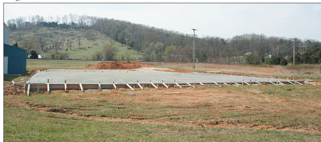
A portion of the concrete slab for a 10,000 square foot warehouse addition to FPL Door Locks and Hardware was poured this week. The company, which is re-locating from California could be open by as early as August.
