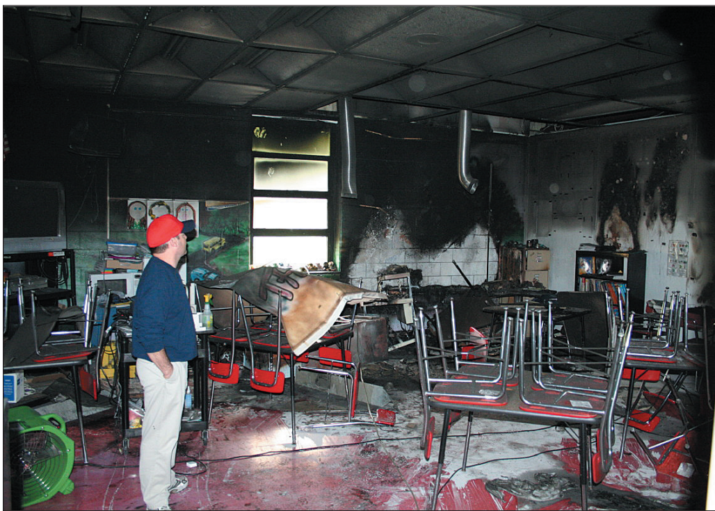
Rockcastle Middle School Principal Jason Coguer surveys the damage to the classroom where Friday morning's fire was started. School officials have estimated that cleanup and repair of the school building could cost as much as $2 million. (Fire photos by Richard Anderkin)
