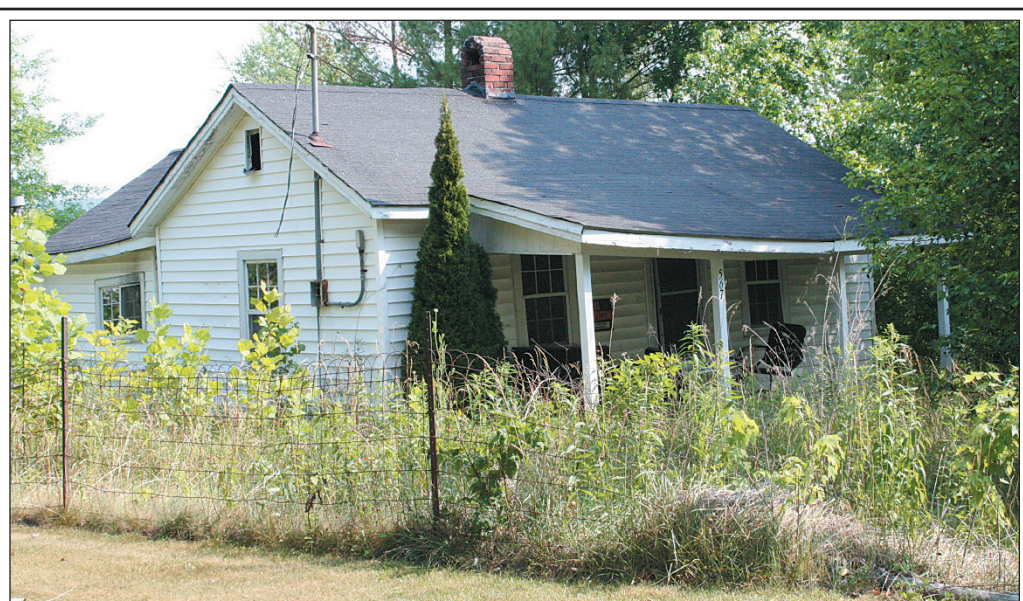
Randy Cromer and his father, Carlis, want the above abandoned house on West Street in Brodhead cleaned up or torn down. The Cromers say the condition of the property is causing a health hazard.
