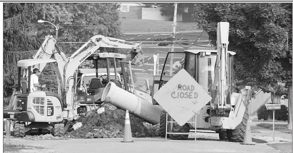
Workers were busy Tuesday putting a 24 inch drainage tile under Newcomb Avenue in Mt. Vernon. The work is part of a $100,000 storm drainage project.
