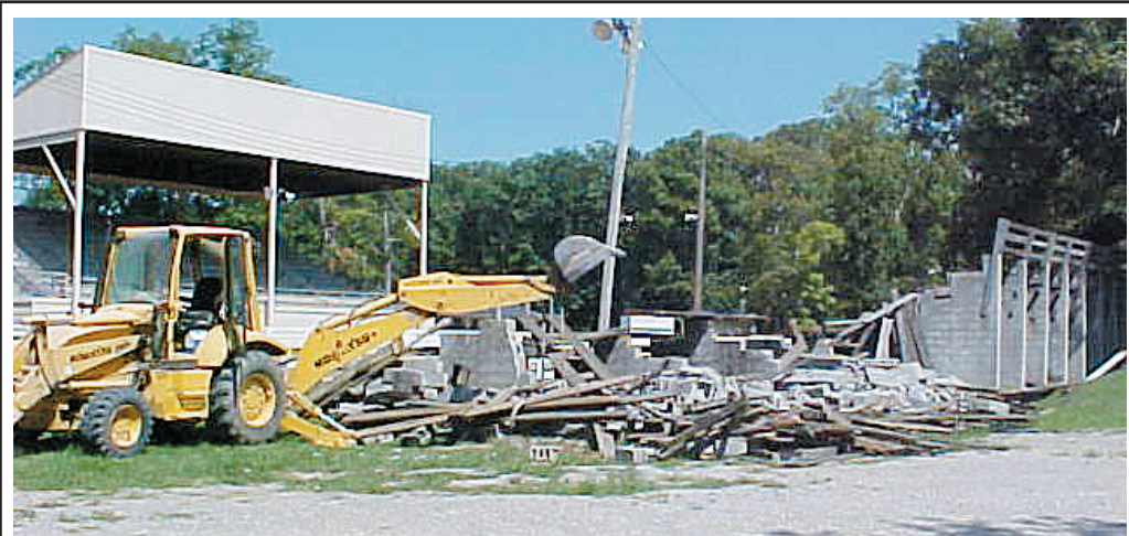
Rockcastle County Road Department employees tore down half of the old bleachers at the Rockcastle County Fairgrounds in Brodhead last Wednesday. The county will apply for a grant, along with the local fair board, to replace the bleachers, which had become unusable. The Little World's Fair is going on in Brodhead this week.
