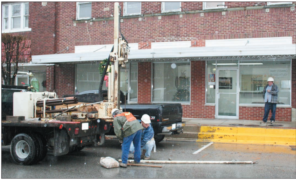
Employees with Hinkle Environmental Services, who work for the state, were in Mt. Vernon again last week taking core samples from land around Dr. John Parsons' building on Main Street. For quite sometime, gas which apparently leaked from old storage tanks left in the ground above Parsons' office, has made its way into his office building, causing an extreme odor and health hazard. The local dentist said the most recent drilling was done to see just how large the perimeter holding the gas underground is.
